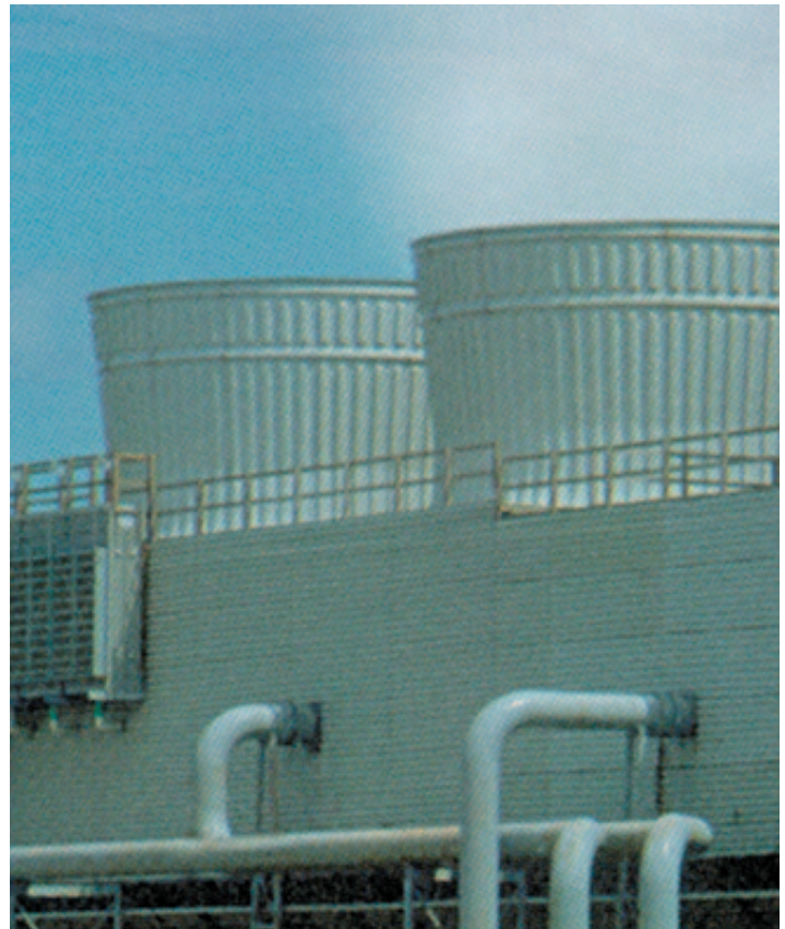
FIGURE 1. No discernible cloud is emitted by the plume-abated cooling tower shown on the left compared to the plumes emerging from the non-abated towers on the right.
